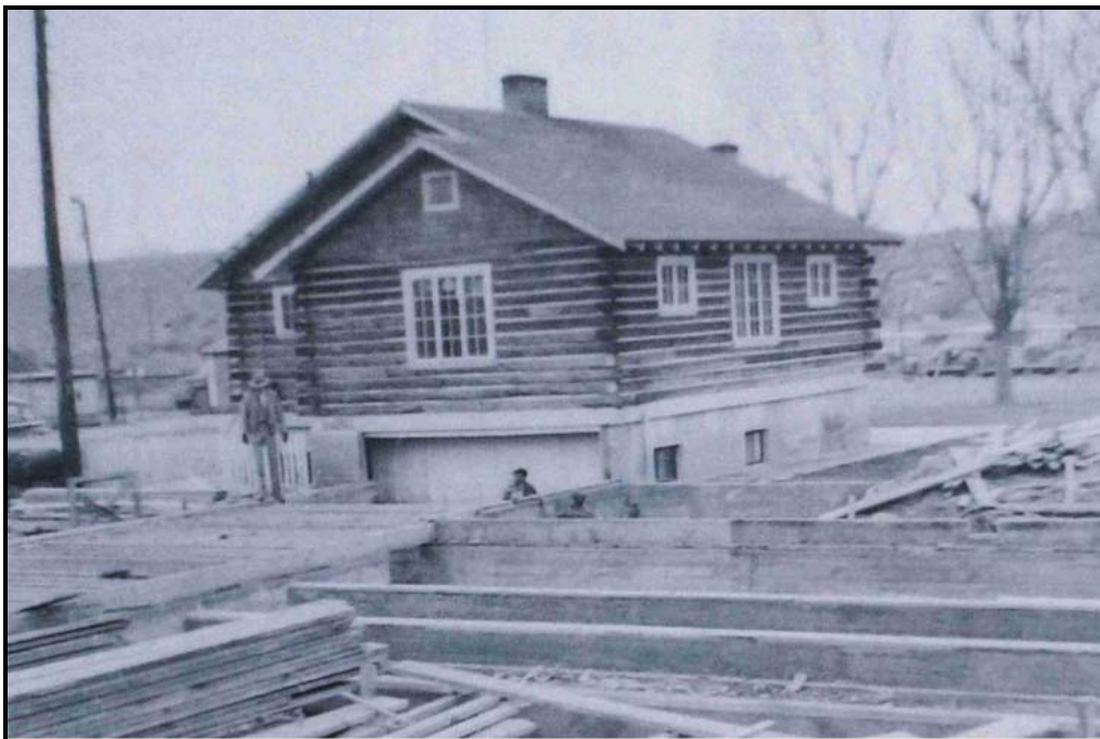
Historic Photo 2. 1948 photograph showing the construction of Building 12 adjacent to the log cabin office. Note the raised foundation of the cabin with the garage entry on the western side. Photographer unknown, on file at the DOE Grand Junction Office, Grand Junction, Colorado.
