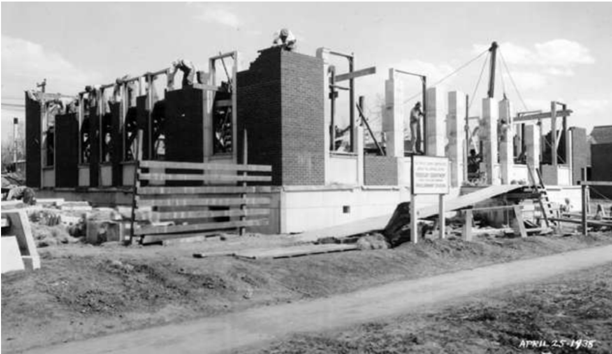
H5: The Englewood Post Office under construction, April 25, 1938. (Source: Denver Public Library, Western History Collection, Digital Photo Collection.)
