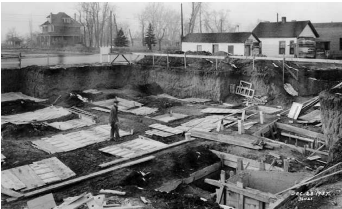
H4: Building concrete forms for the Englewood Post Office foundation, December 23, 1937. (Source: Denver Public Library, Western History Collection, Digital Photo Collection.)
