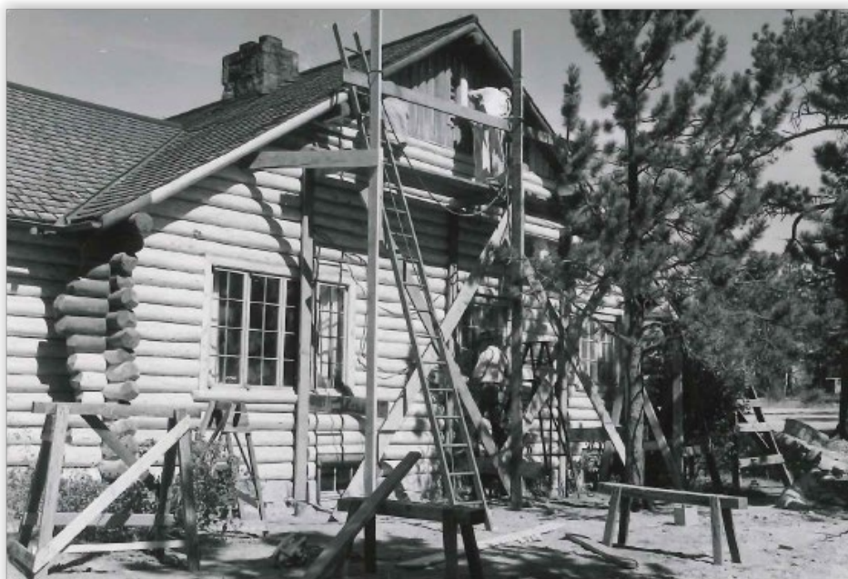
Figure 15: Forest Carpenter Mirl Boner (right) and Fire Guard Glenn Scott (left) refinishing the Ranger Dwelling in 1954. Note refinishing work underway on the log crowns to the left. Source:
