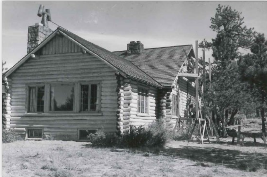
Figure 14: Work underway on the Ranger Dwelling refinishing project in 1954. Scaffolding is on the southeast gable. Photograph by E.H. Mason, Forest Supervisor. Source: Roosevelt National Forest Scrapbook, on file at the Arapaho and Roosevelt National Forests and Pawnee National Grassland Forest Supervisor's Office, Fort Collins, CO.
