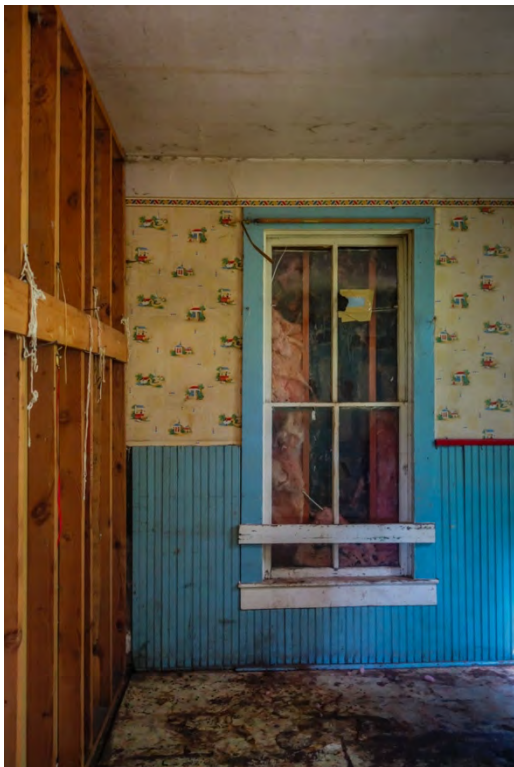
Photo 44 • Glassier House, main floor interior. Image shows original exterior window enclosed by frame addition. Looking northwest, June 2017 – (unchanged as of 2023)
