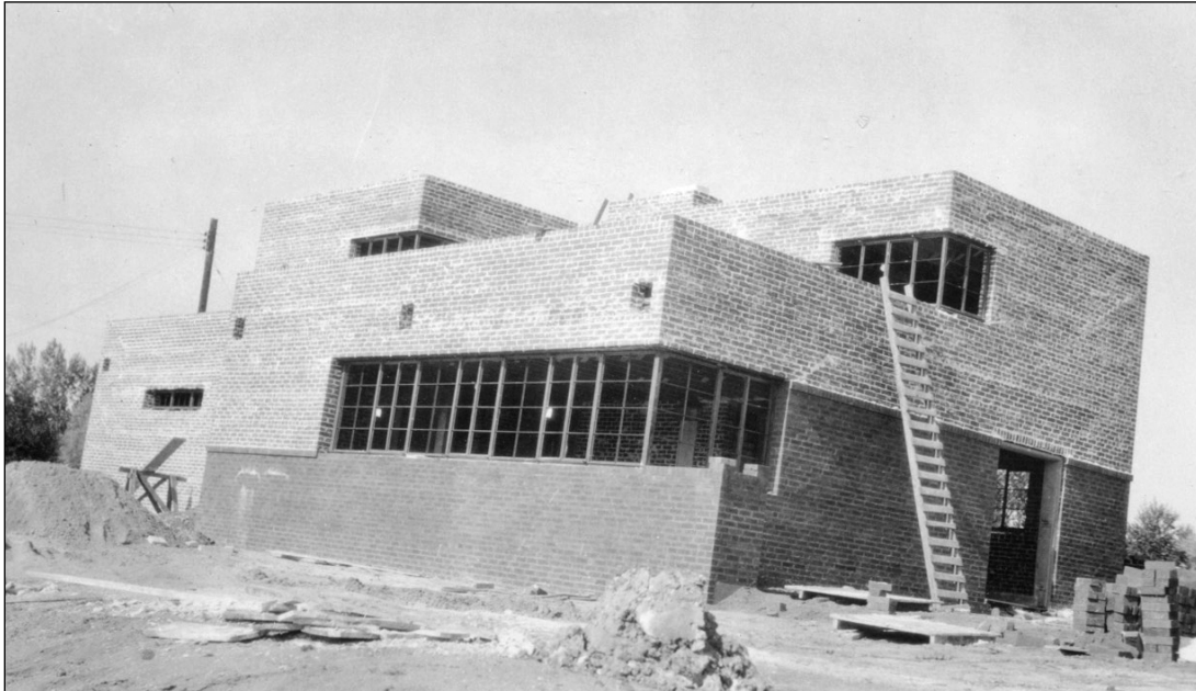
Figure 4. This 1935 construction photograph (view northwest) shows the completed brick walls and the installed steel casement windows. SOURCE: Frank Hegner photograph collection, on file Carol and Tom Amy, Denver, Colorado.
