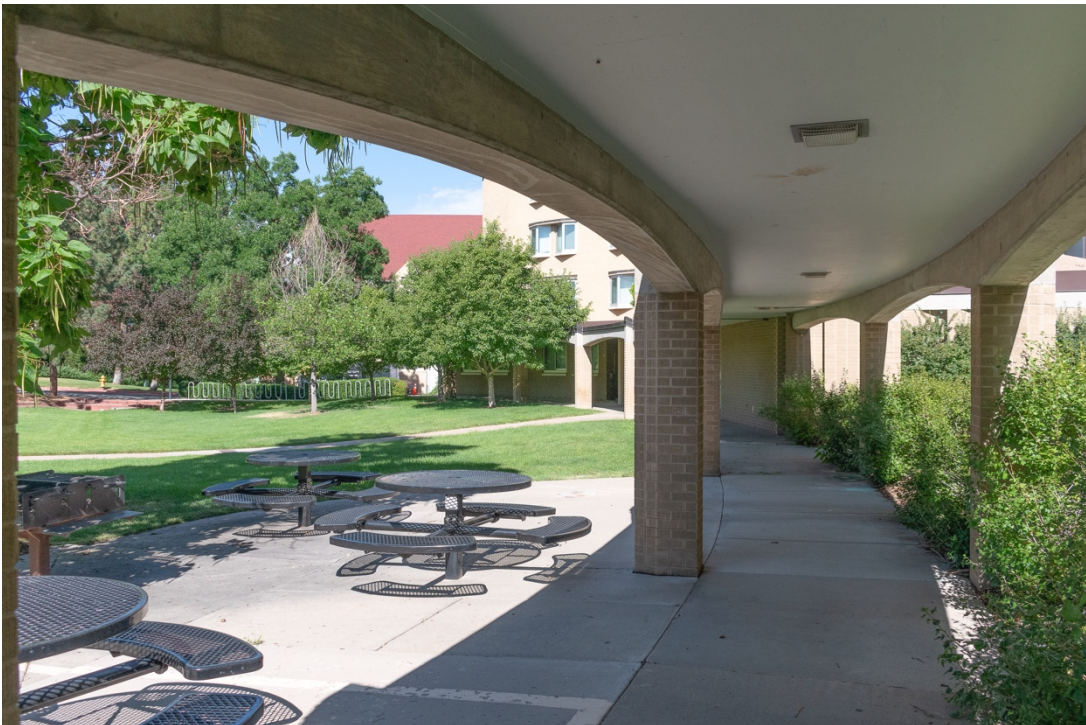
CO_Denver_CWC_0044: Dunklee Hall, east end of walkway on south elevation, facing west
