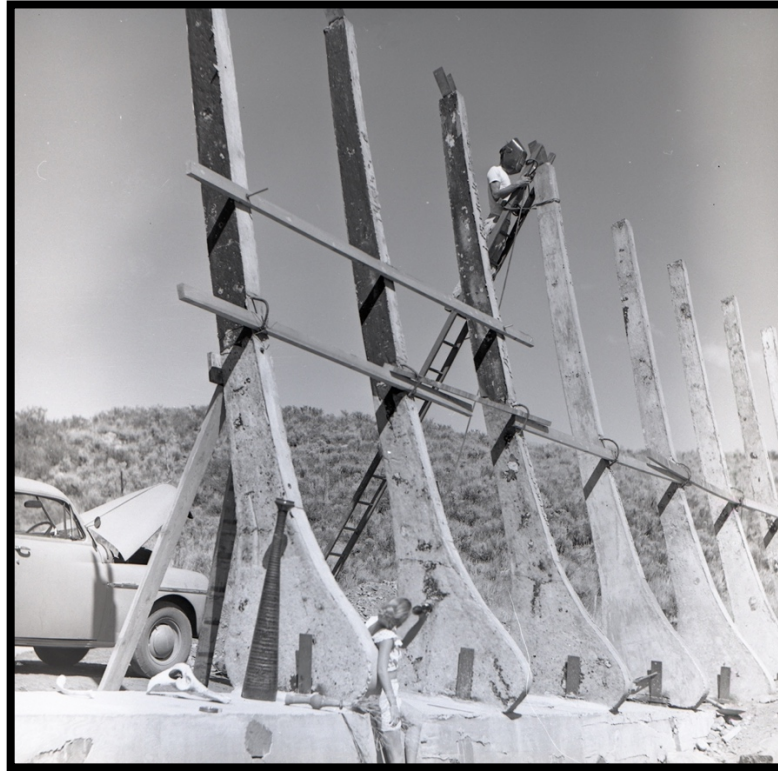
Photo 13: Erecting the A-Frame Building, 1960. From the Collection of the Soldner Family Partnership LLLP.
