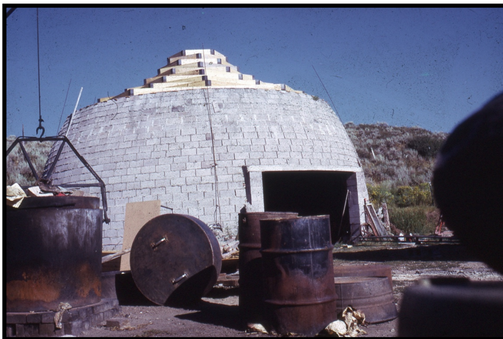
Photo 16: Round Building Under Construction, circa 1969. From the Collection of the Soldner Family Partnership LLLP.
