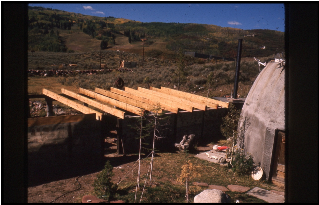
Photo 18: The Studio Building (Long Building) Under Construction, 1974. From the Collection of the Soldner Family Partnership LLLP.
