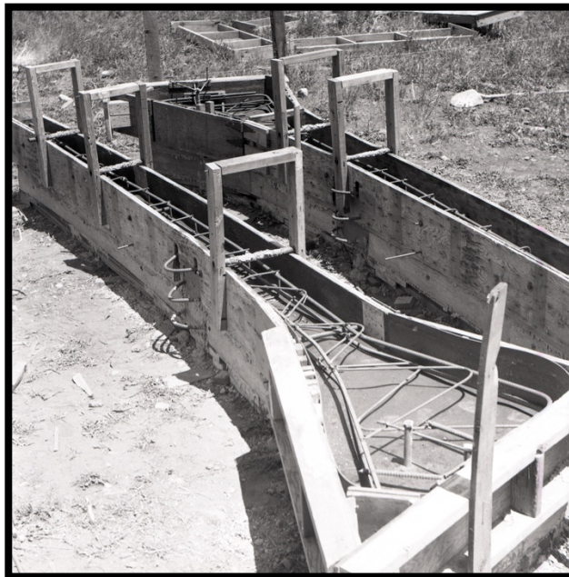
Photo 12: Cast Concrete Beam Frames, A-Frame Building, 1959. From the Collection of the Soldner Family Partnership LLLP.
