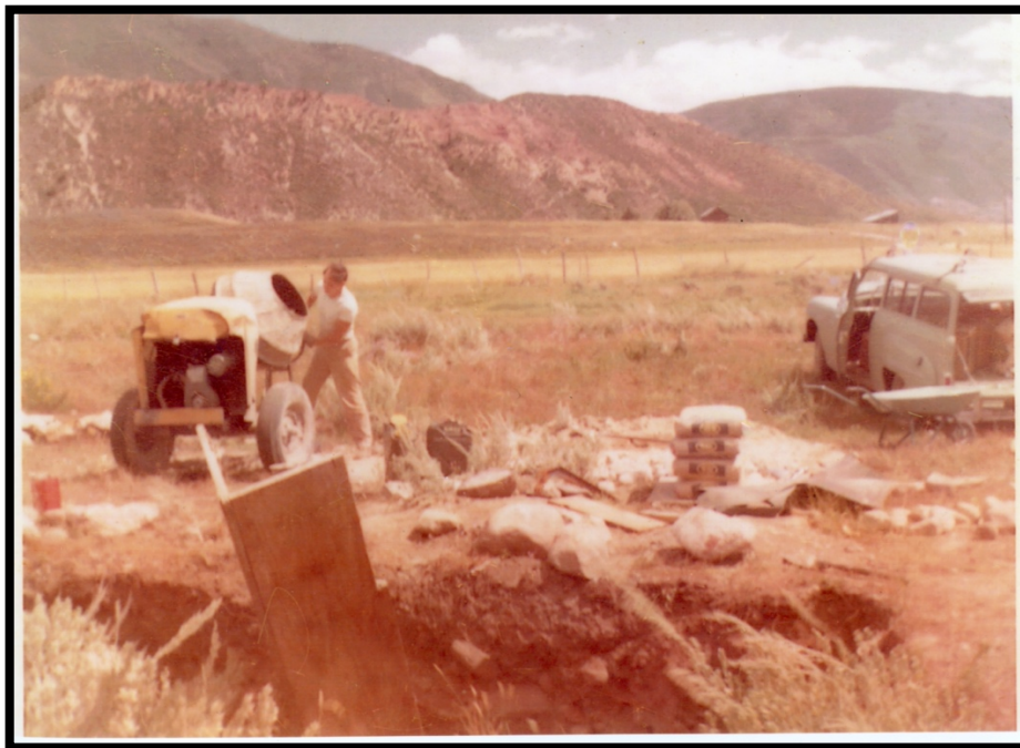
Photo 6: Paul Soldner Mixing Cement on the Site, circa 1958. View to the East. From the Collection of the Soldner Family Partnership LLLP.
