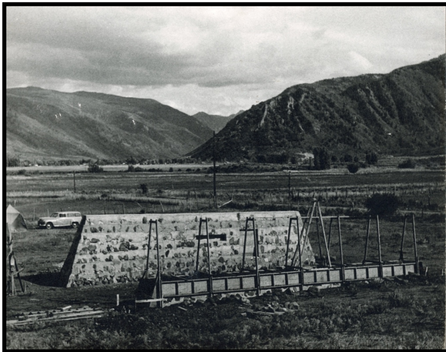
Photo 9: Orange Door Building Under Construction, 1958. View to the East. From the Collection of the Soldner Family Partnership LLLP.
