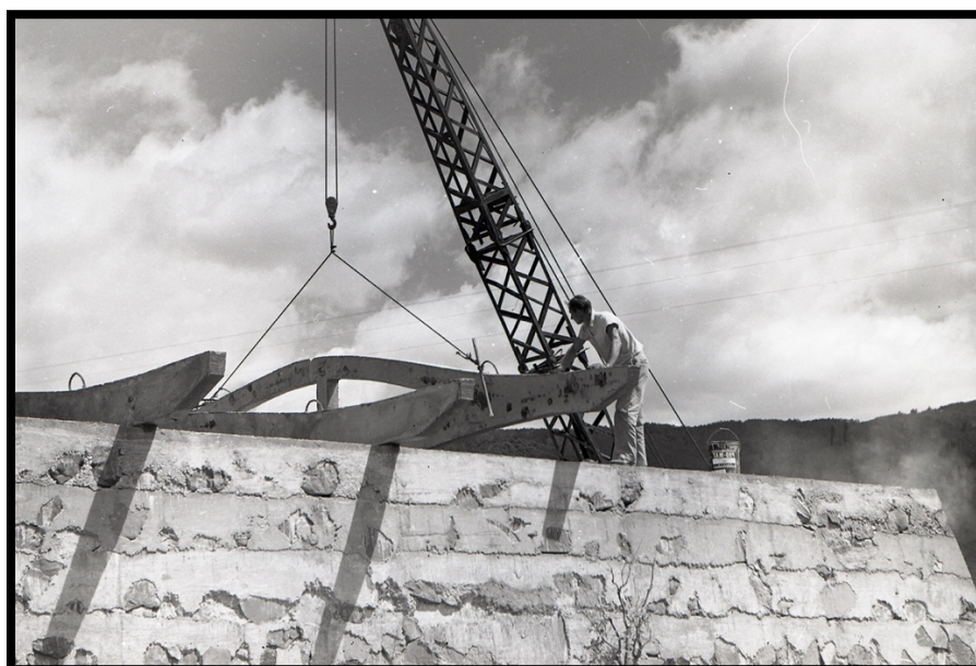
Photo 10: Orange Door Building, 1959. Paul Soldner Guiding Roof Beam into Place. From the Collection of the Soldner Family Partnership LLLP.
