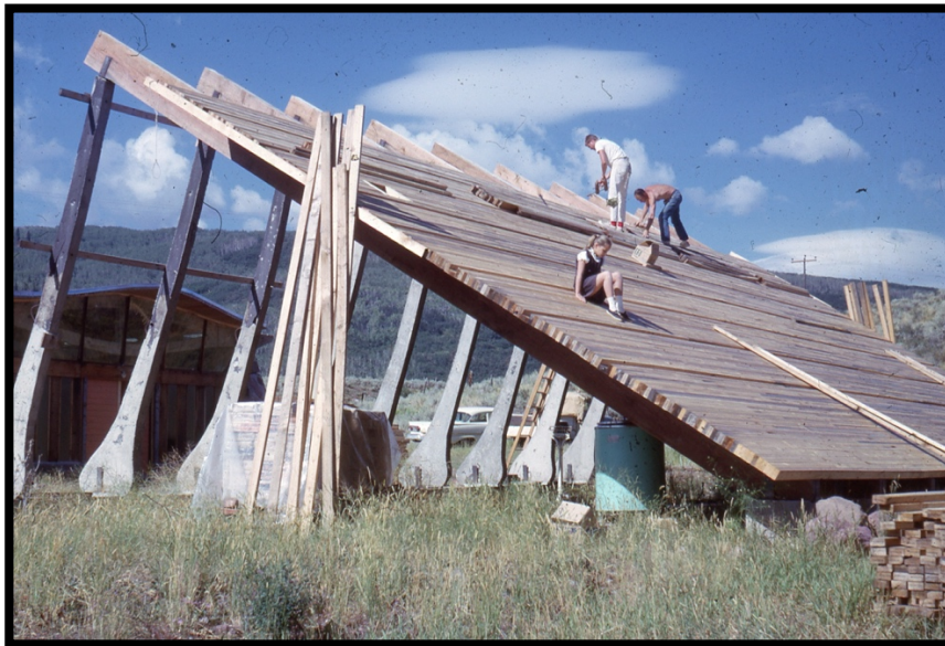
Photo 14: Erecting the A-Frame Building, 1962. From the Collection of the Soldner Family Partnership LLLP.
