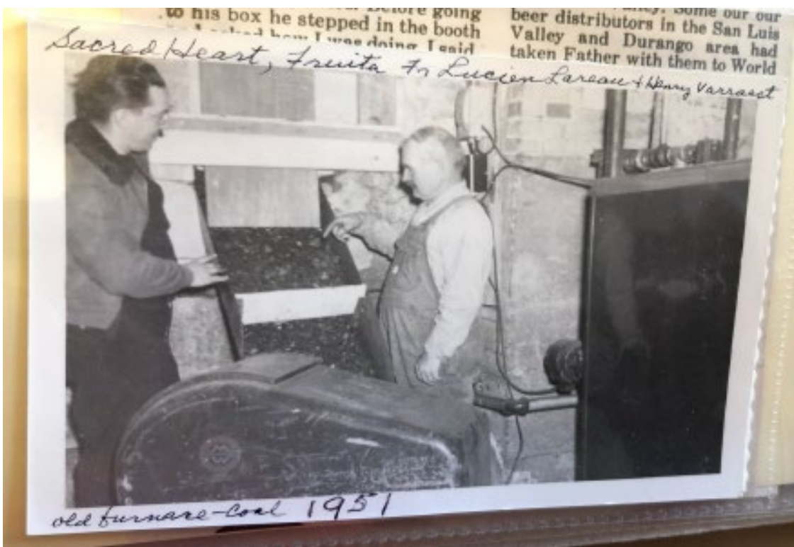
Photo H4. Photo of coal-fired furnace and boiler located in basement, at base of chimney, ca. 1951.
