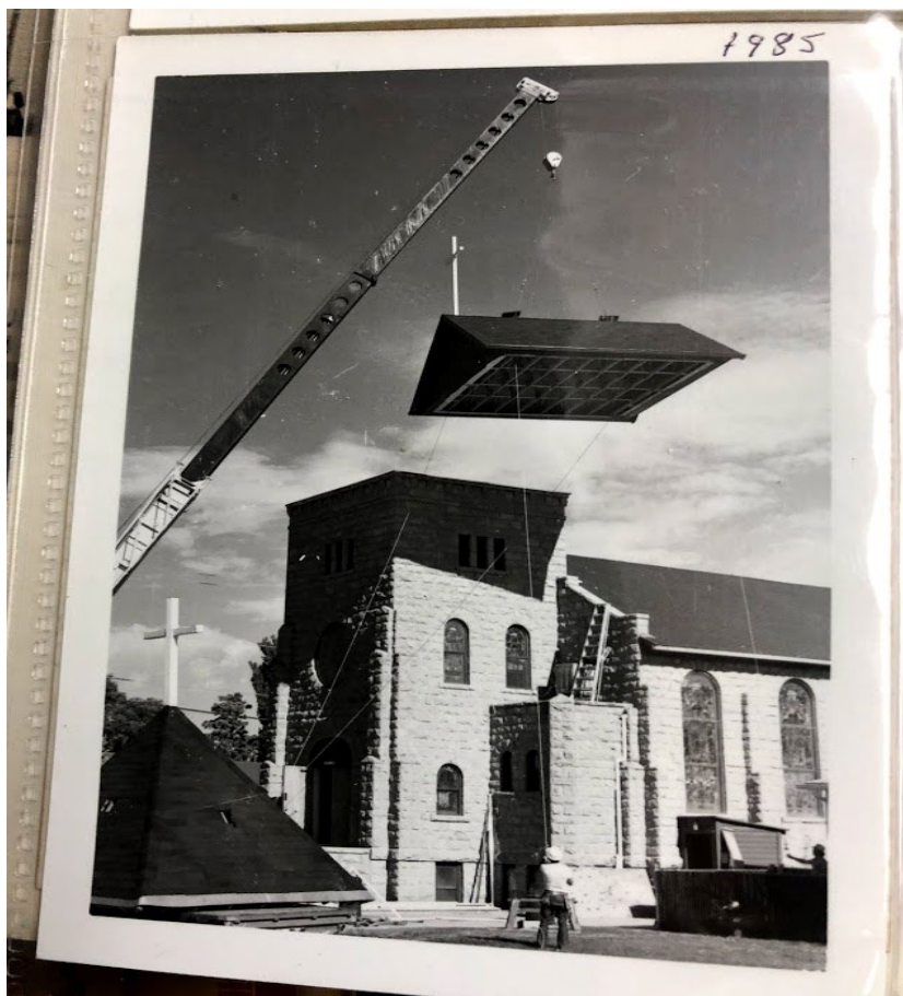
Photo H7. Replacement of bell tower roof, ca. 1985. Original roof structure in left foreground.
