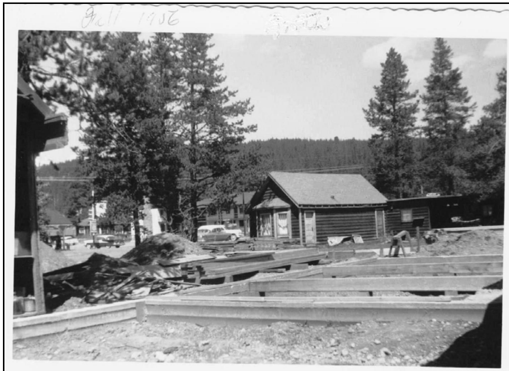
Figure 13. Photo of three-unit cottage court-type building under construction on Smith-Eslick property, Fall 1956
