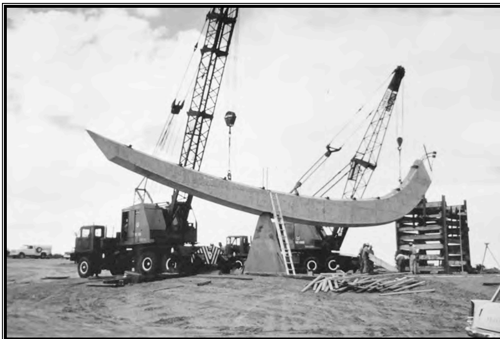
HP-1: Lifting the First Roof Beam into Place, October 1963 (Courtesy of Joel Haertling)
