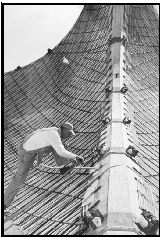
HP-3: Attaching and Tightening the Catenary Cables, January 1964 (Courtesy of Joel Haertling)
